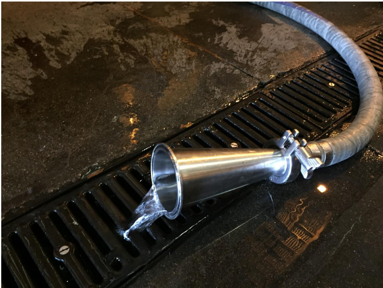
Figure 11. Unmetered water use. Winemakers are more concerned about making a good wine than worry about conserving water. One winery removed internal water meters used to calculate their water use outside of other commercial use within the winery. Photo by author.
