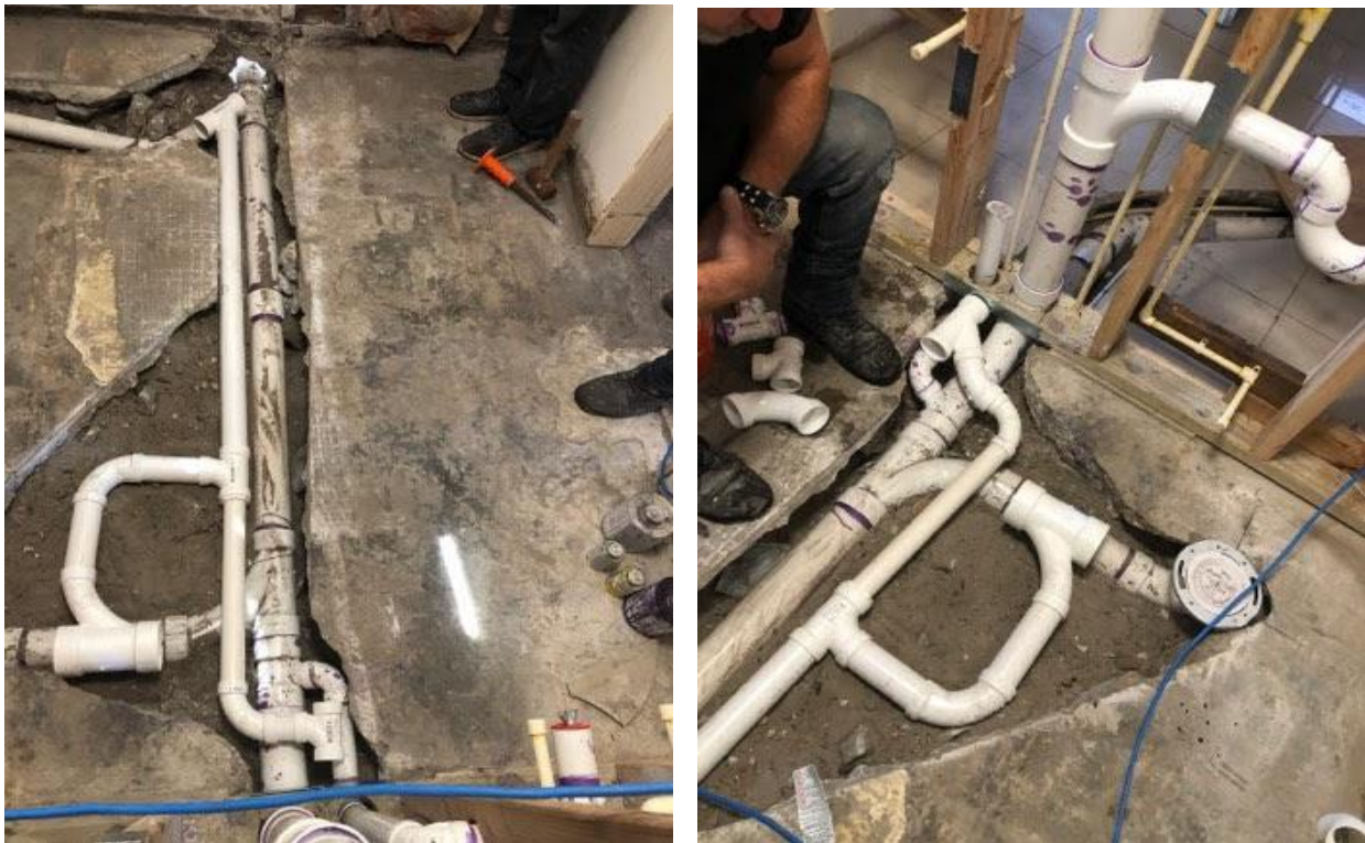
Figure 11: Maria and Manuela’s DIY plumbing project. The first layout (left) was not approved because the pipe bends for the toilet, shower, bathroom sink and kitchen were too close. Following advice from the inspectors, their refined layout (Right) was approved (Photos by the participant).
