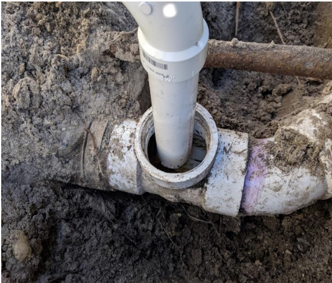
Figure 10: A Master bathroom sewer pipe connecting to the new-laid sewer pipes that carried sewerage to the city's main sewer line (Author).
