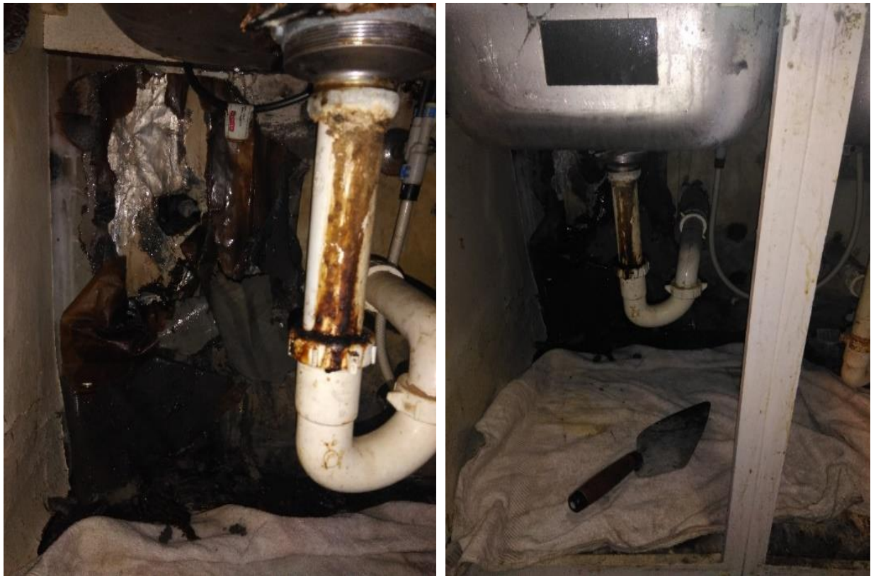
Figure 8: Pictures that were taken by Stacey and family during a sewer backup incident in May 2019 (Photo by the participant).
