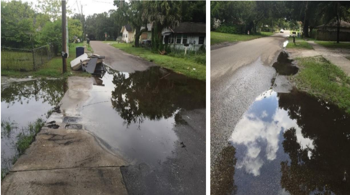
Figure 15: A pool of water between empty plots at Site 3 (left) and small water pools at Site 2 (Right) (Author).
