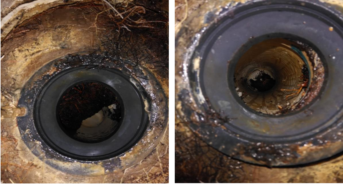
Figure 9: Tree roots growing in sewer pipes at Stacey’s house (Photo by the participant).
