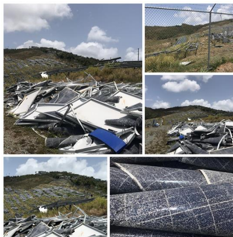
Figure 47. Donoe Solar Array After Irma & Maria 2017 (Photo Credit: Maya Trotz, July 2018)
