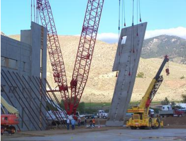
Figure 1: Tilt-slab construction requires careful consideration of the center of mass (source – intmath.com )
