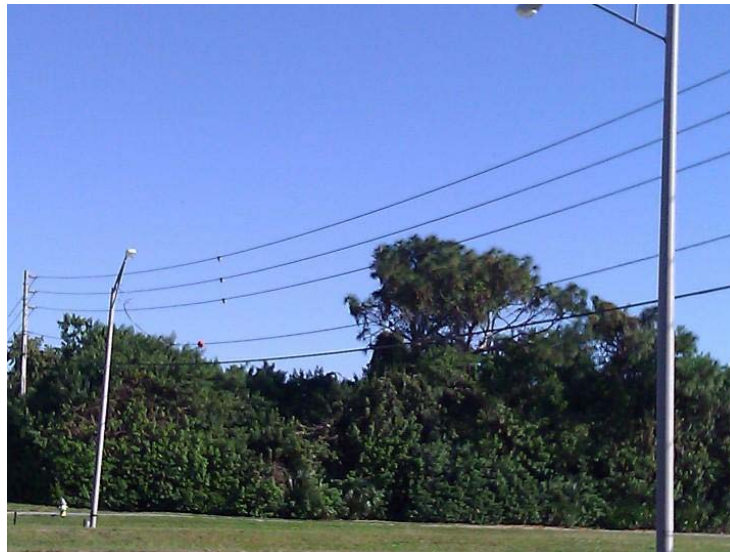
Figure 1: A cable hanging between to power poles.
