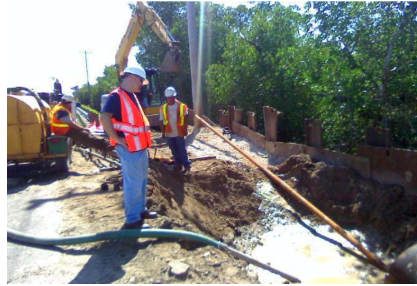
Figure 3: At the exit hole workers are placing a larger diameter reamer to widen the hole to fit the pipe.
