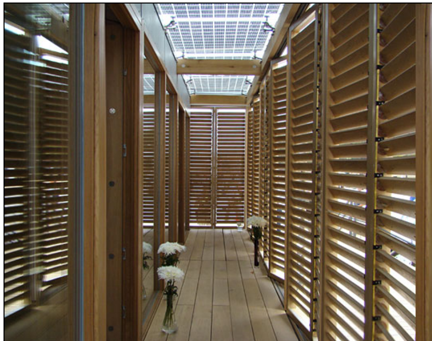
Fig.25 Louvers are closed to provide shade and protect actual walls and glazing from heat gain.
