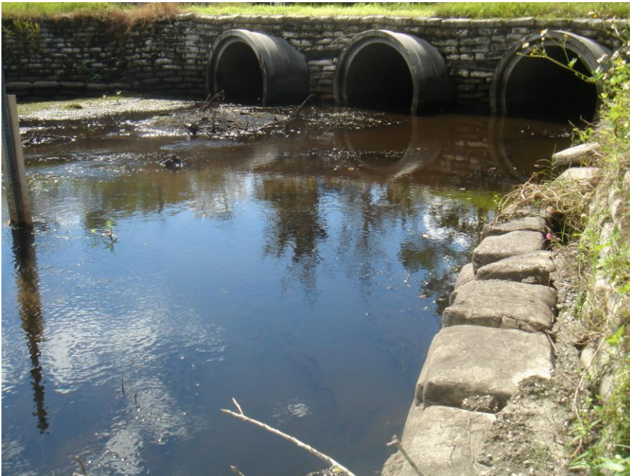
A-8. Upstream sampling site 9/26/2009. Maintenance crews had recently removed sediments and hydrilla from the creek bed.
