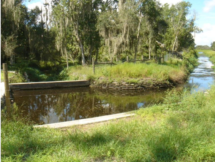
A-9. Diversion structure on the left and canal to Balm Road Treatment Marsh on the right 9/26/2009.
