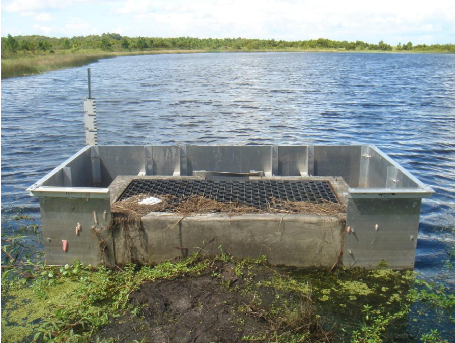
A-11. Treatment system outfall structure in cell #4 9/26/2009.
