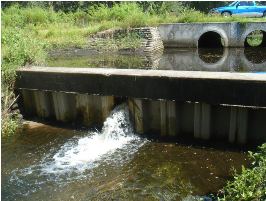
A-10. Diversion structure allowing base flow to Bullfrog Creek 9/26/2009. All additional flows are directed through the canal on the left that flows to Balm Road Marsh.
