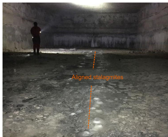
Fig. 7. Stalagmite growth near station CAU-2 aligns with fractures in the gallery's ceiling. This growth pattern strongly suggests that fracture flow is a key characteristic for drips in Caumont Quarry.
