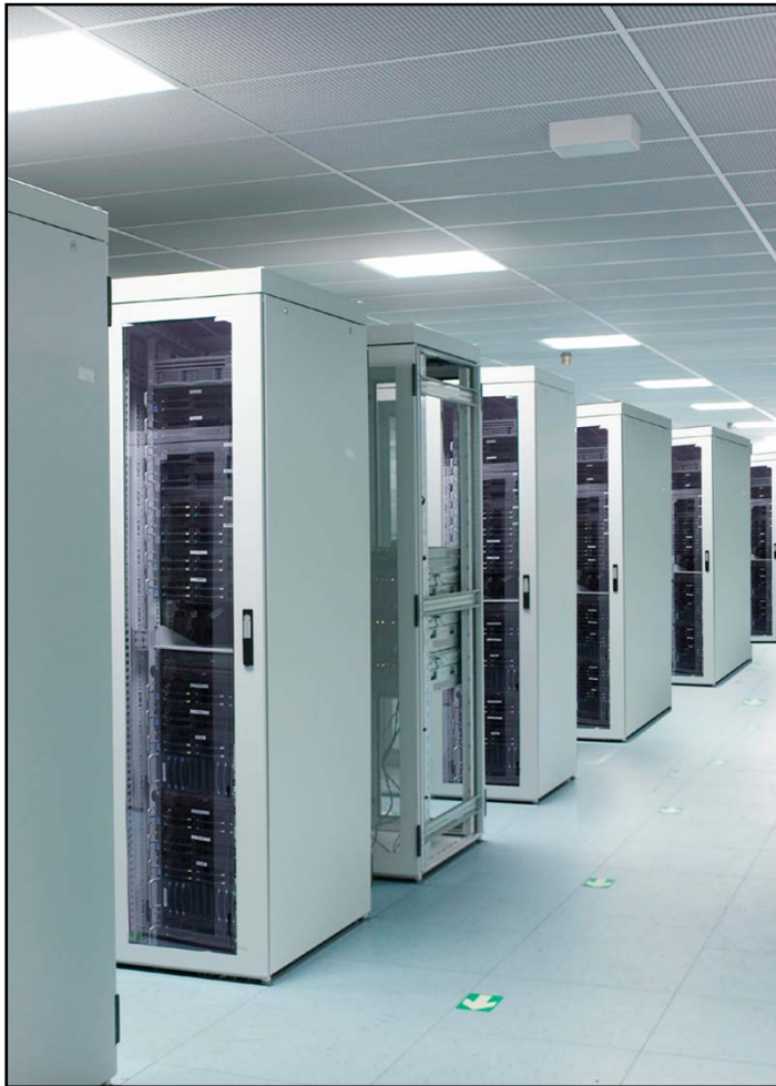
Figure 89: Off-site Computing Warehouse
