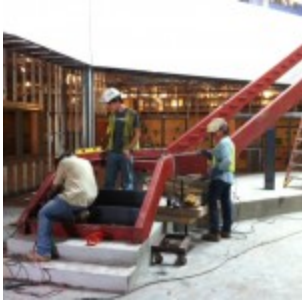
Construction crew works on the grand staircase at the new Student Life Center.
