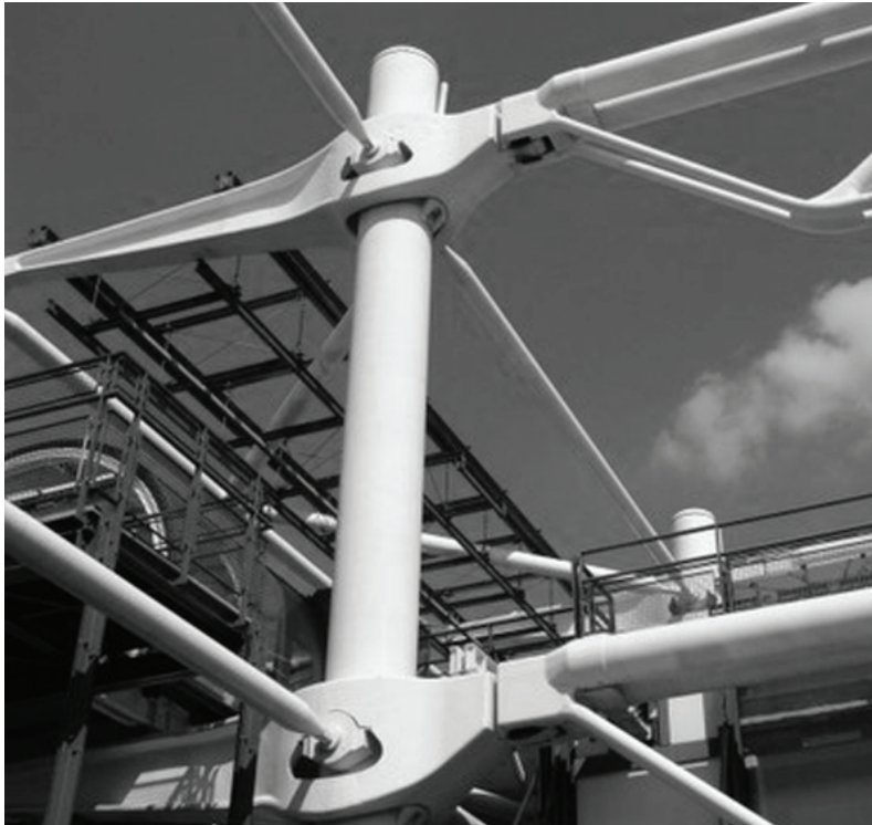
Figure 2.13 structural detail. Silver, Nathan. The Making of Beaubourg : A Building Biography of the Centre Pompidou , Paris. Cambridge, Mass.: MIT Press, 1994.
