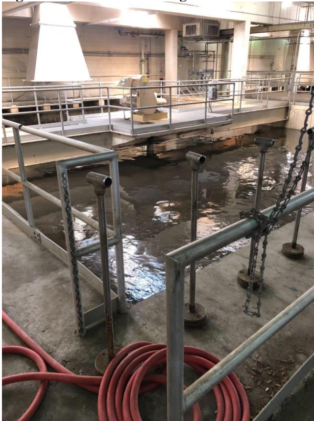
Figure 10. Inside the City of Tampa Water Treatment Facility during interviews
