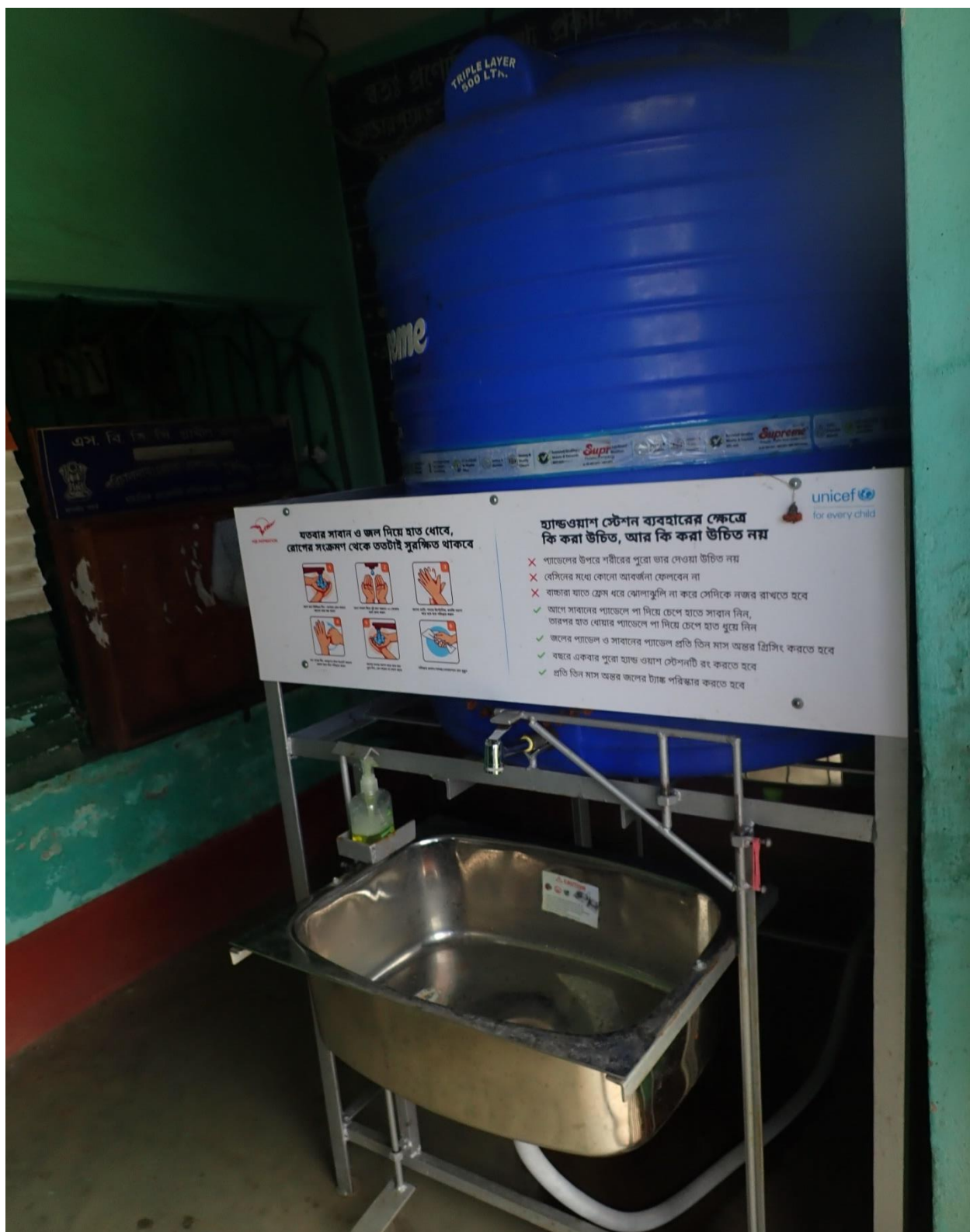
A handwashing station installed in one of the village council offices in Purulia. Participants often also mentioned drinking water from this source.
