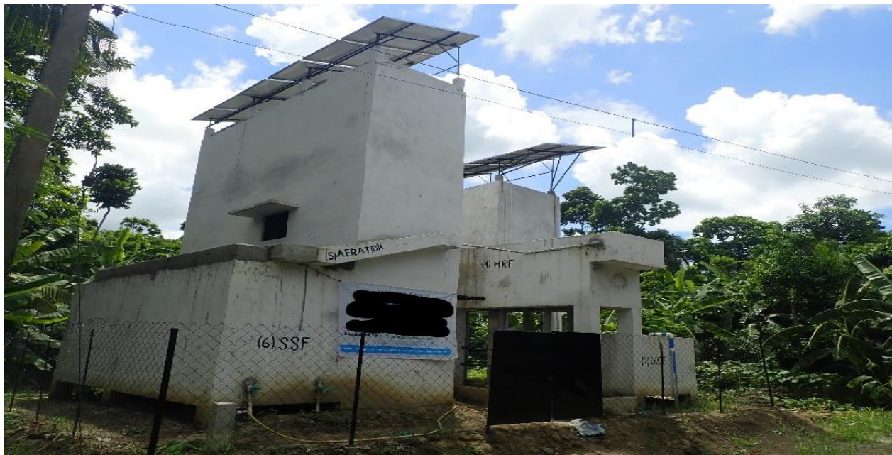
Figure 4. Water Treatment Plant
