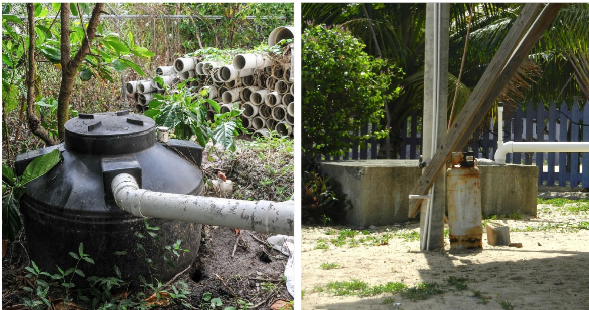
Figure 21. [Right] A plastic tank and [right] a pre-cast cement tank. Photos by EC Wells
