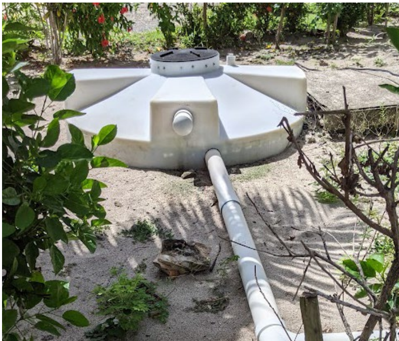
Figure 7. Septic system behind a large office building on the main street. September 2021.
