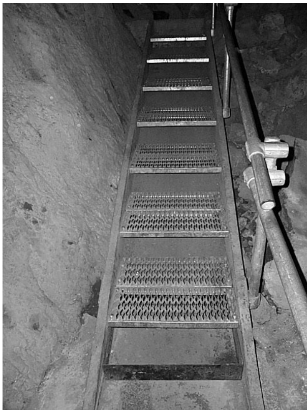
Figure 3. New stairs in Skull Cave made of galvanized steel with \frac{1}{2} -inch mesh. Also notice the steel tray under the structure and catchment trough at the base of the stairs (photo by Kelly Fuhrmann).
