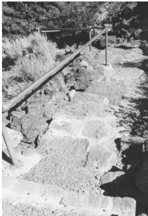
Figure 16. Photograph taken in August of 2000 from the same location as Figure 15. All loose debris was removed, new basalt lava slabs added, and the trailhead renovated. (Photo by Kelly Fuhrmann)
