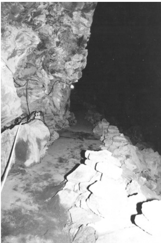
Figure 12. A basalt sand base was added over the original trail tread material. (Photo by Kelly Fuhrmann)
