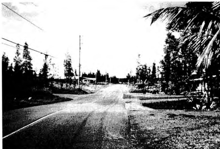
Figure 1. View looking up hill on Ainaloa Boulevard, one of the few paved streets in the Puna subdivisions. The dip seen near the center of the photo resulted from sagging of the street into the partially filled entrance of Lower Uilani Cave during road construction. The skylight is just to the right of the light- and dark-colored surfaces. Underlying the light-colored surface and part of the road is a dump of household and automotive solid wastes, partially in plastic nonbiodegradable bags. (Photo by W.R. Halliday)
