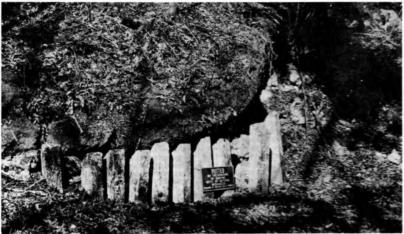
b. Second entrance: original gate (like the one shown above including concrete blocking) already restricted bat and air movement. Concrete posts, added later, almost totally closed the entrance. Uninformative signs such as these probably do little to engage the cooperation of cavers.
