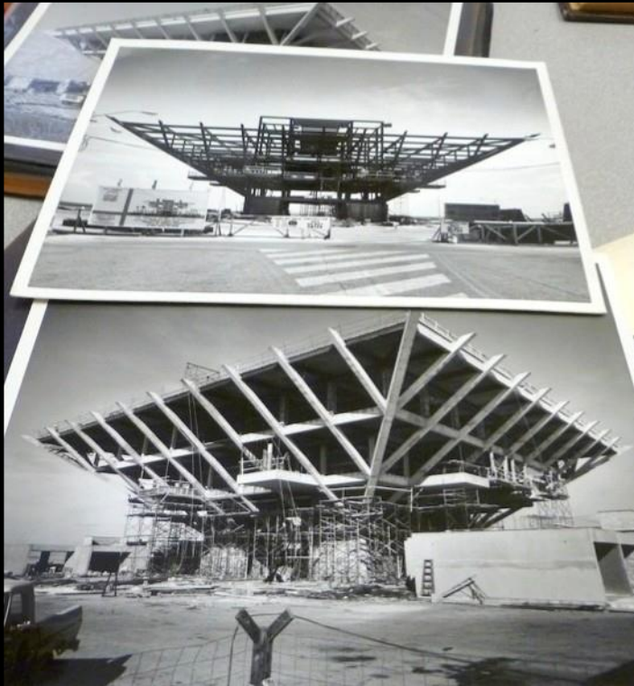
Figure 46. The Pier Under Construction (Photo Courtesy of Archives of Harvard Jolly Architecture).
