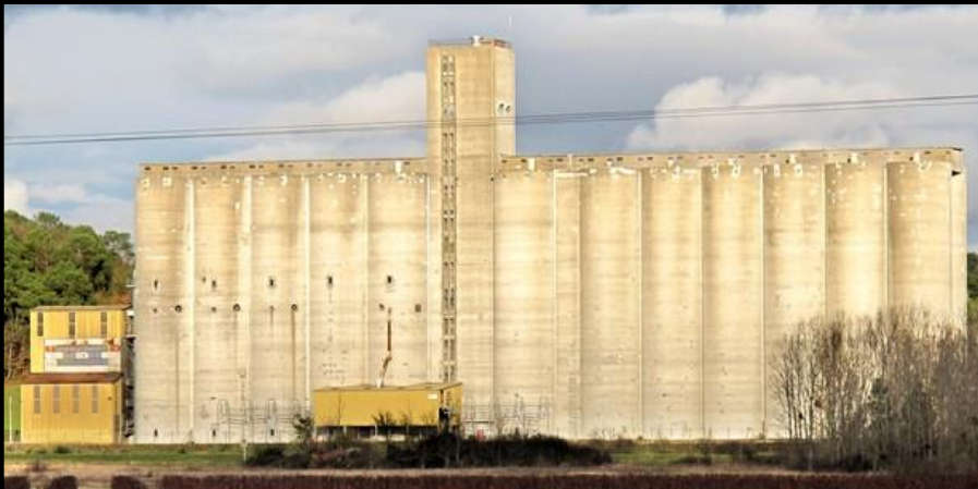
Figure 15. Cylindrical Silos in Saint-Romain-sur-Cher (Photo by Daniel Jolivet; Creative Commons License, http://bit.ly/1fXjo6q ).
