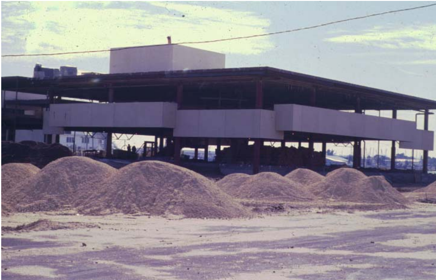
A view of the original Nelson Poynter Memorial Library, now Bayboro Hall, during construction in 1980.
